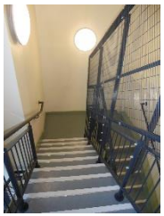
Handrails not continuous with the landings
